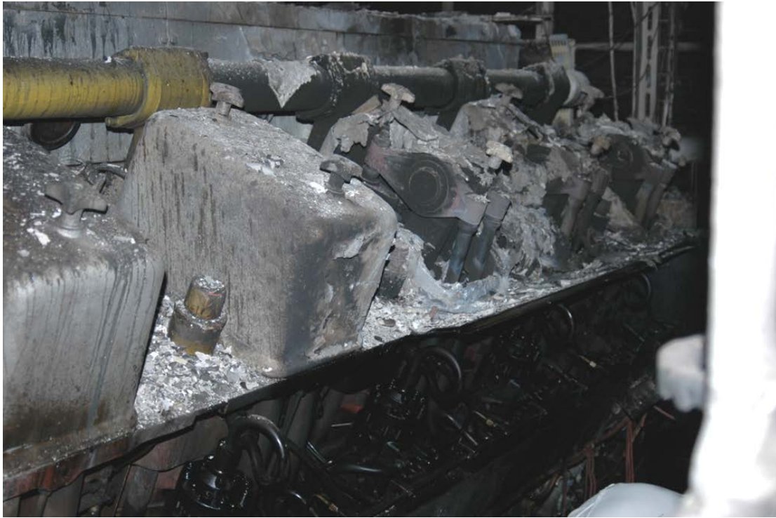
Engine No. 4 post fire looking forward on the inboard side towards the seat of the main fire. The hot box cover has been removed in this view and it is possible to see the fuel piping and the injector pumps for each unit.
