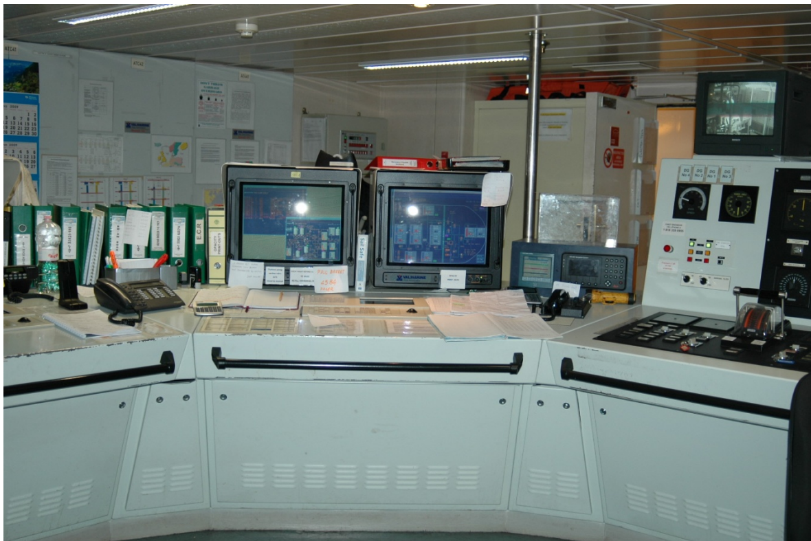
ECR control panel looking forward towards the port side showing (centre of picture) the position for the watch engineer and to the right the central part of the panel which has the engine controls. Above the engine controls can be seen the first screen of the camera monitoring system.
