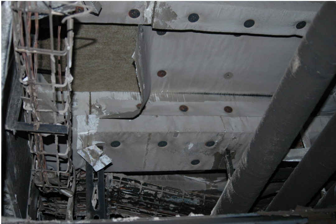
View of the engine room deckhead above the fire showing fire insulation intact and secured with only minor damage to covering material. Note cable trays with the cables completely burnt away.
