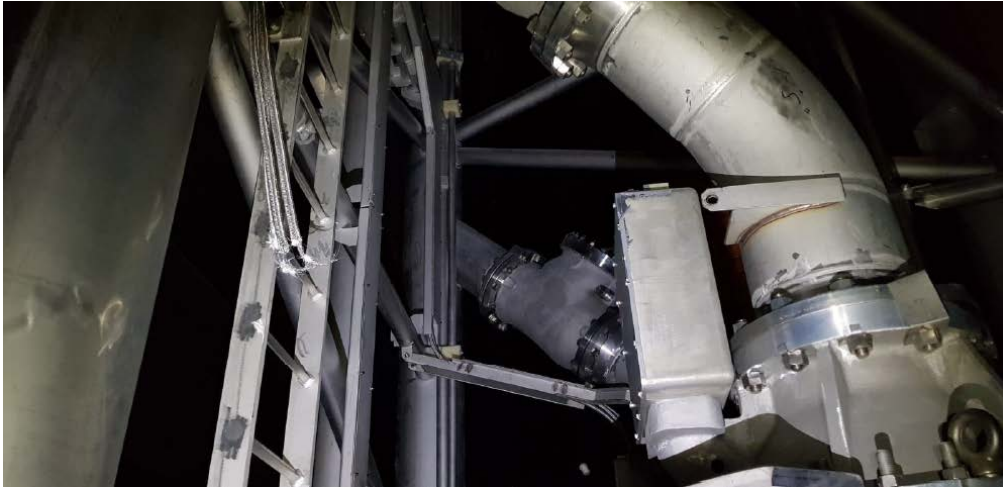
Fig. 1: Location of fallen cable tray
